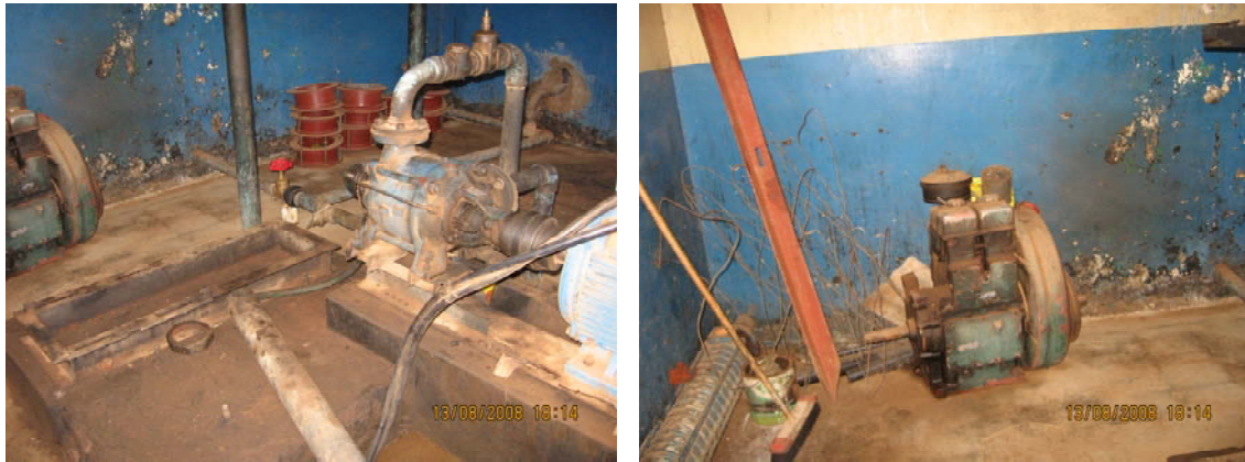
Plate 9: Bondo Water Booster Station
