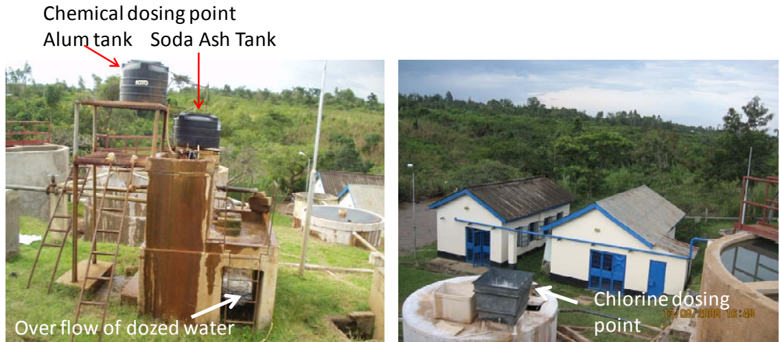
Plate 5: Chemical dosing points
