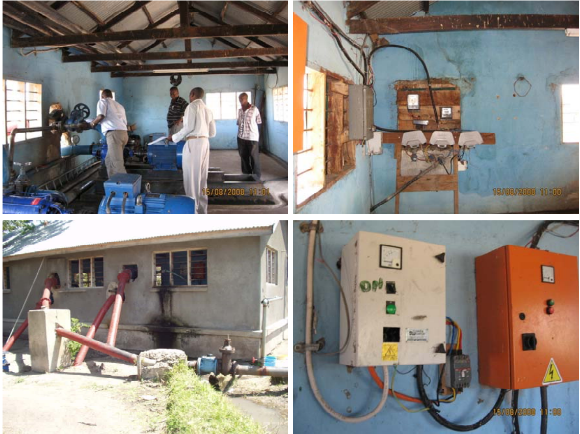
Plate 16: Raw water pumps and electrical panel units at Gupta pumping station
